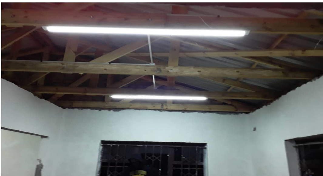
After wiring the hostel and installing the solar system which is working with a 5KVA inverter, lights are now functioning.
